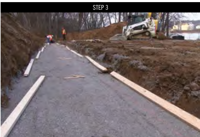
Forming up to pour a 2" unreinforced concrete overlay for setting the first course of Mega-Tandem™ (MSRW). A 6" crushed stone leveling pad is an option as well.
